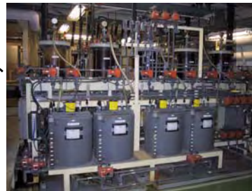
MRT Plant for Rhodium Recovery
