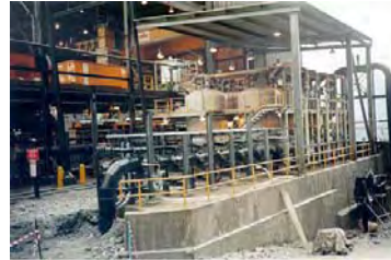
MRT Plant for Acid Mine Drainage Treatment
